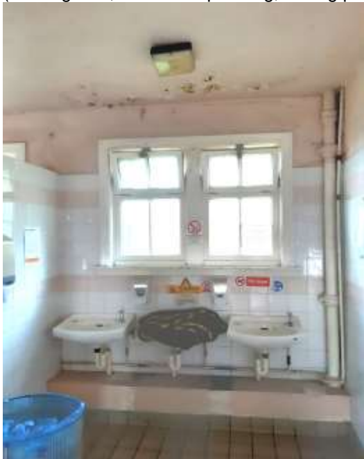
Photo 3. Interior (Ladies) (missing sink, towels in open bag, flaking paint)
