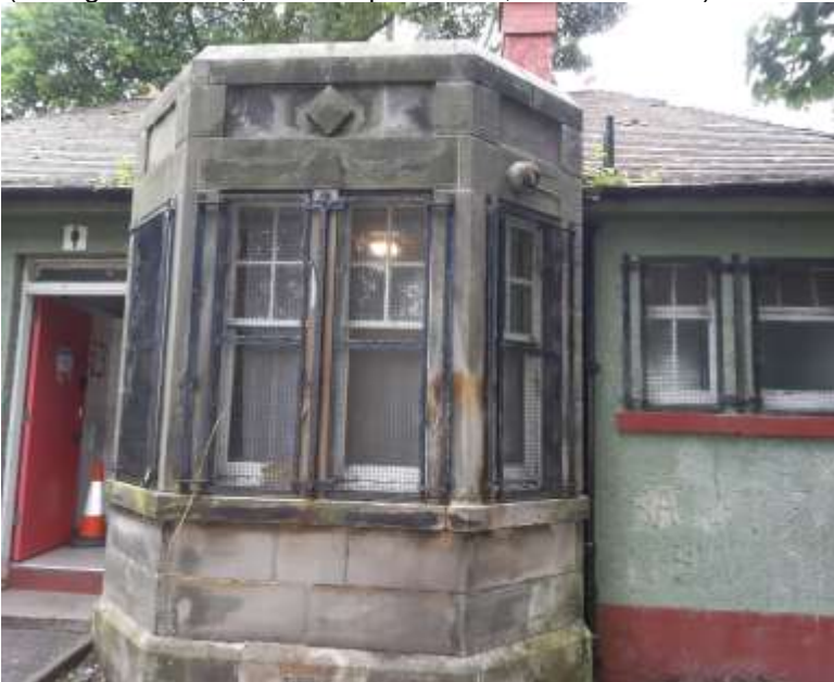
Photo 1. 'Welcome' to Cramond's Toilets (flaking stonework, fenced-up windows, weeds on roof)
