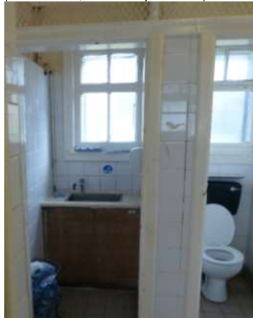
Photo 4. Interior (Gents) (no hot water, boarded up sink unit)
