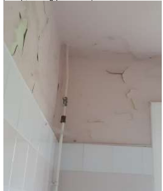
Photo 2. Interior (Ladies) (damp, flaking paintwork)
